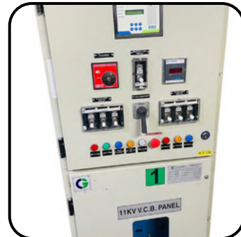
VCB Panel Alarm
