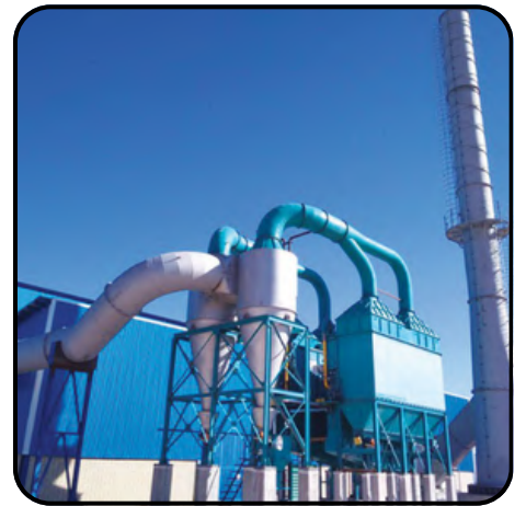
Air Pollution Control System
